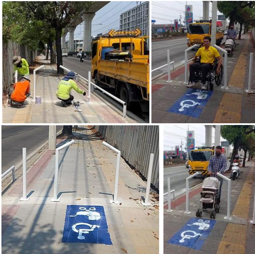
Figure 5 Installation and testing for wheelchair and baby stroller.
