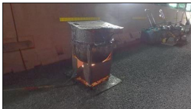
Figure 5. Melted waterproofing material by gas burner.
