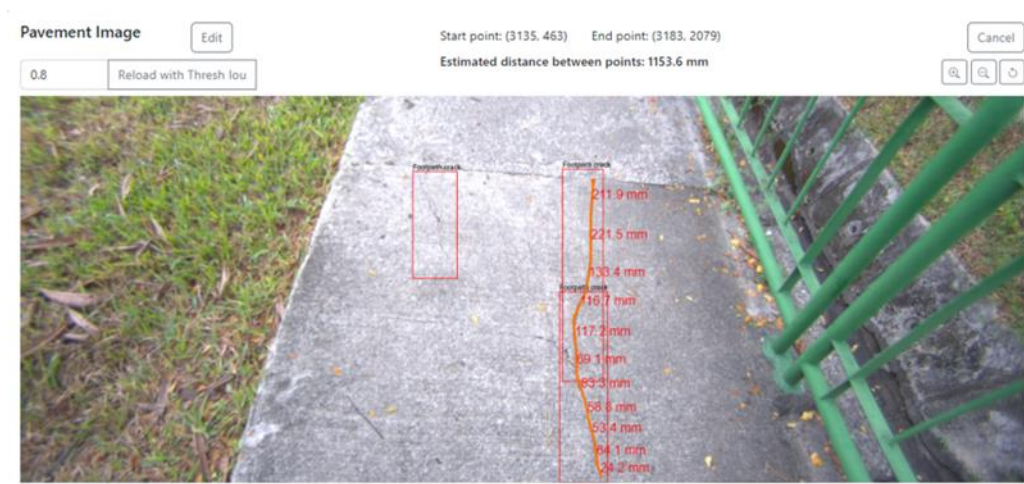
Figure 6 Image of pavement containing crack defects with estimation of the crack length.
